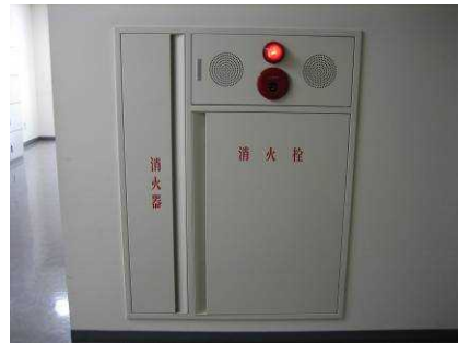
Fire alarm (top) and hydrant (bottom)
